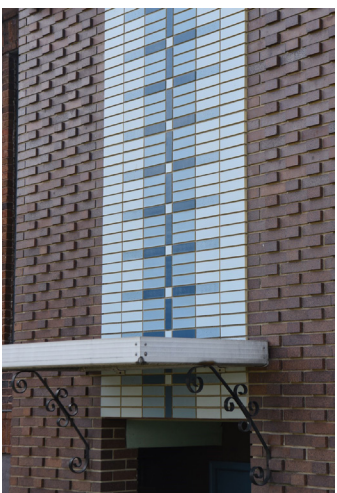
Fig. 15. Wall fragment from the Holy Cross Church in Dayton (OH), 1964, architect Jonas Mulokas [from authors private archive]
